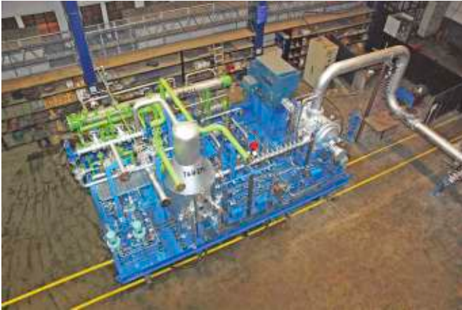
Gas Compressor Package in a Refinery
